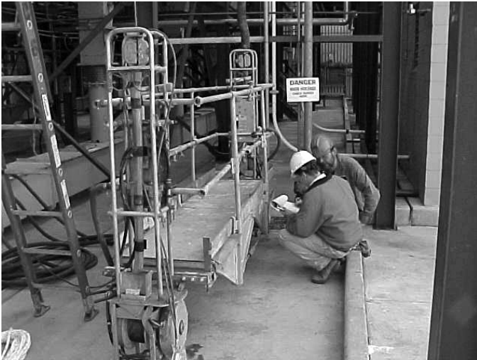
ST-26 attached to platforms
